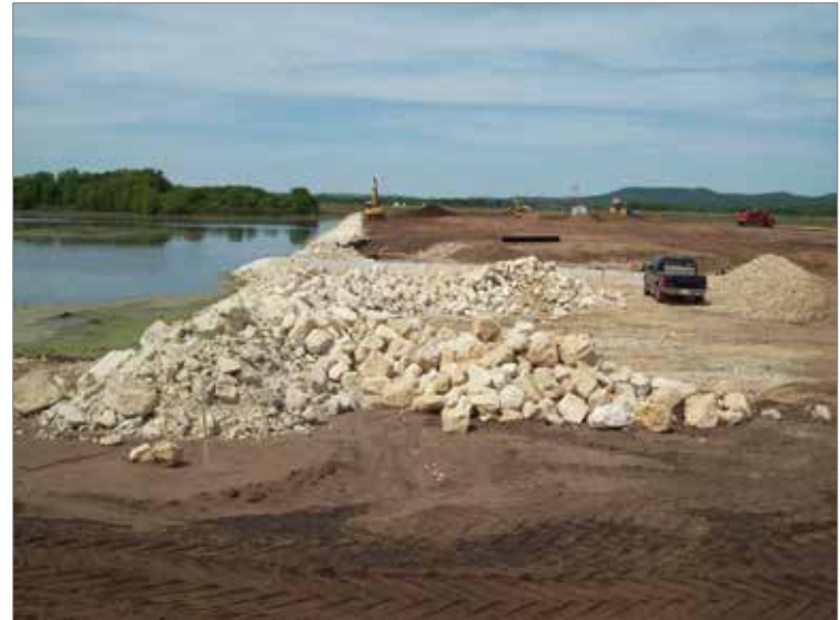
Fill requiring 404 permit and mitigation
