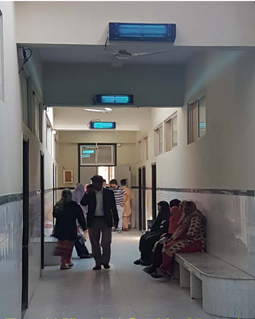
Karachi Hospital Corridor Natural Ventilation UVGI + Fan
