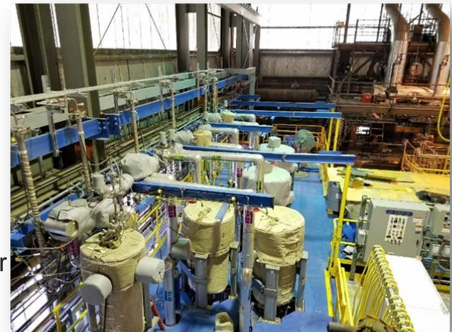
METL Facility , Argonne National Laboratory
